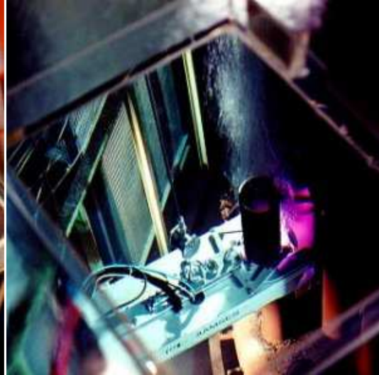
Figure 14. The plasma cutting device during segmenting the stand pipes (the cutting time for each pipe using a 100 A plasma torch was approximately 1 minute)
